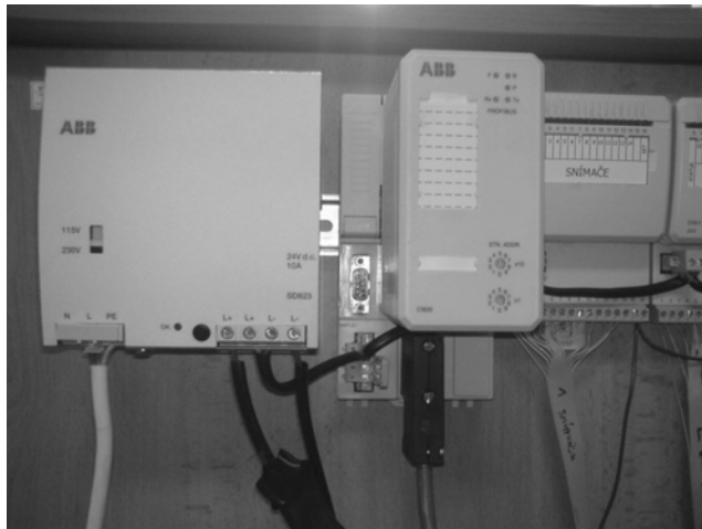
Fig. 3 Power supply, ProfiBus and I/O modules
