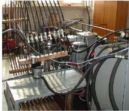
Fig. 4 View on the measured device
